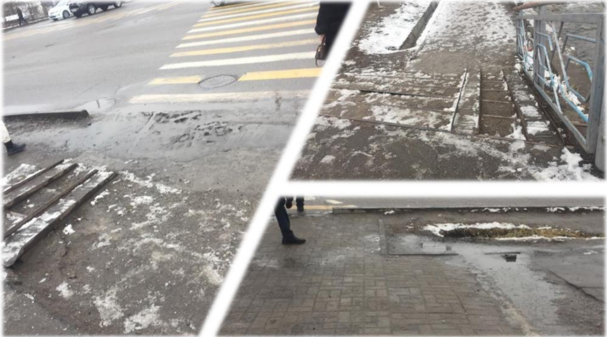
Figure 2: Adjacent sidewalks, stairs, ramps of crossroad at Maldybaev – Akhunbaev location before upgrades
